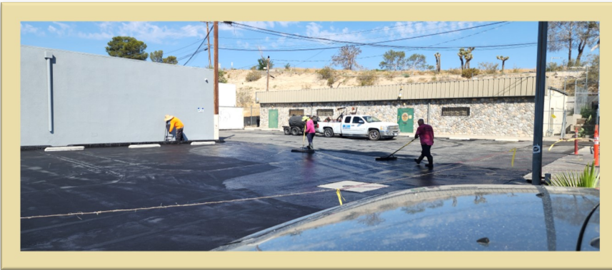
The grading crew hard at it to produce a bright, new parking lot.
